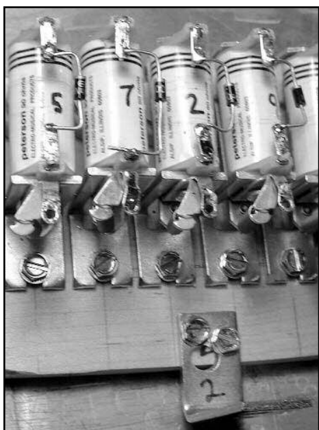
Figure 31. Diodes installed on the valve coils, with broken lug. Note the white polarity mark at the ends.
